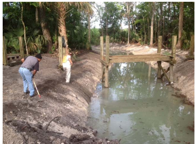
Photo No. 2 – Newly dug canal and boardwalk between Central Park Lake North and the adjacent lake to the east
